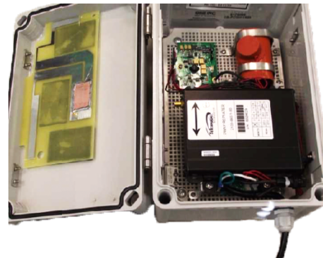
Figure 2: Allegro AC-Powered Repeater ( internal photo )
