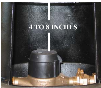
Distance between pit lid and meter
